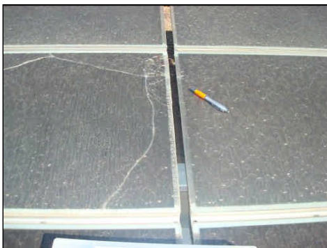
“Goat damaged” First Solar laminate
